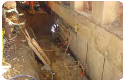
Above: The biggest challenge faced by both the contractors ... was that the Odlins building was older, bigger, wetter and more rotten than most.
