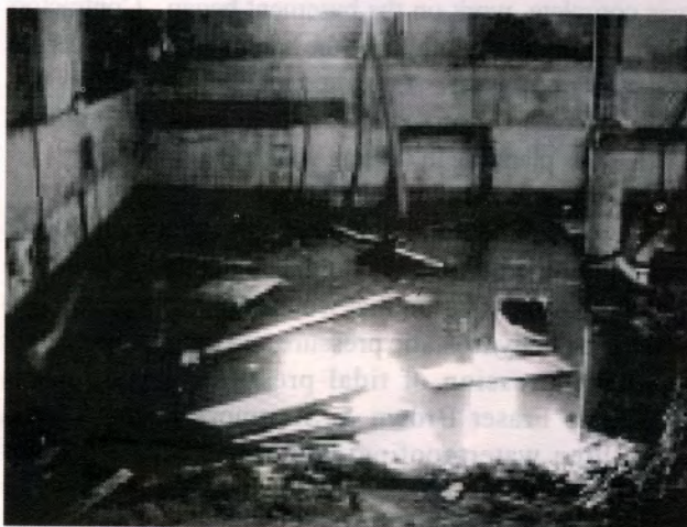
Above: Contractors were literally swimming since the basement was submerged under 1.5m of water.
