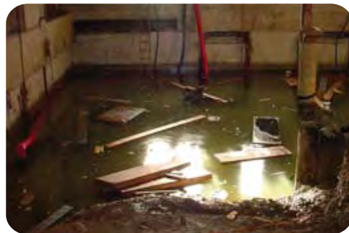
Below: Contractors were literally swimming since the basement was submerged under 1.5m of water.
